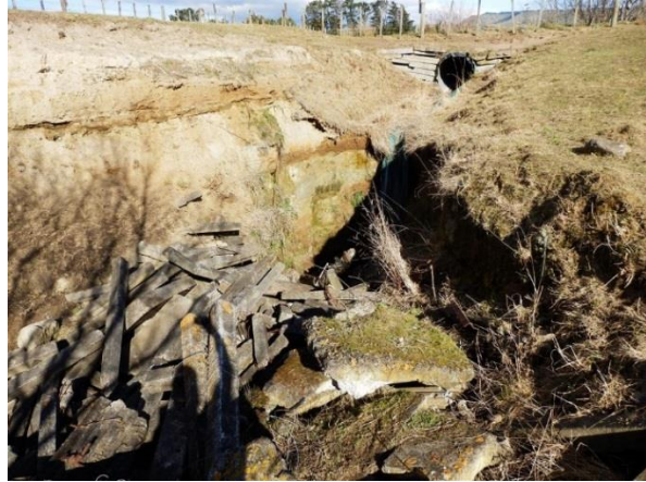
Fig. 8 Gully head erosion at poorly stabilised farm dam outlet; extensive repair is required, including a suitably designed flume.
