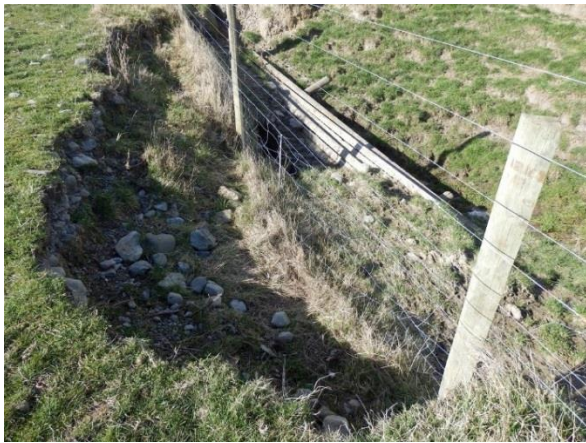
Fig. 7 Erosion of crossing embankment by overtopping flow; culvert pipe requires design size check and a high flow Spillway should be installed.
