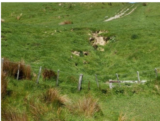
Fig.1 Track runoff point and erosion on culvert embankment, no runoff controls in place.
