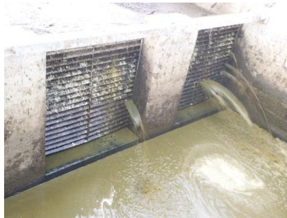
C. Weeping wall in collecting pond
